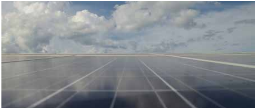
View of solar panels in Scatec's Los Prados solar power plant
